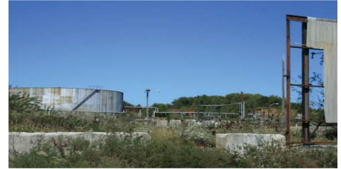
Storage tanks are in the process of being removed at the former Farmland property
