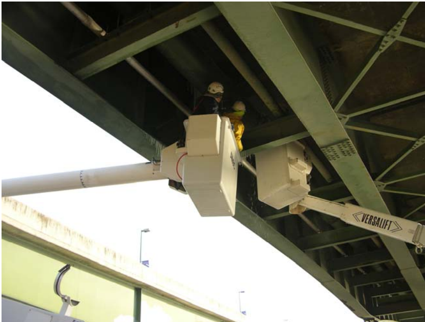
At left: Water distribution crew inspects a leak in the water main under the Kansas River Bridge. Parks and Recreation and Public Works staff assisted with the use of their bucket trucks to repair the leak. Good teamwork and quality staff in this emergency situation helped resulted in no loss of water service to north Lawrence.
