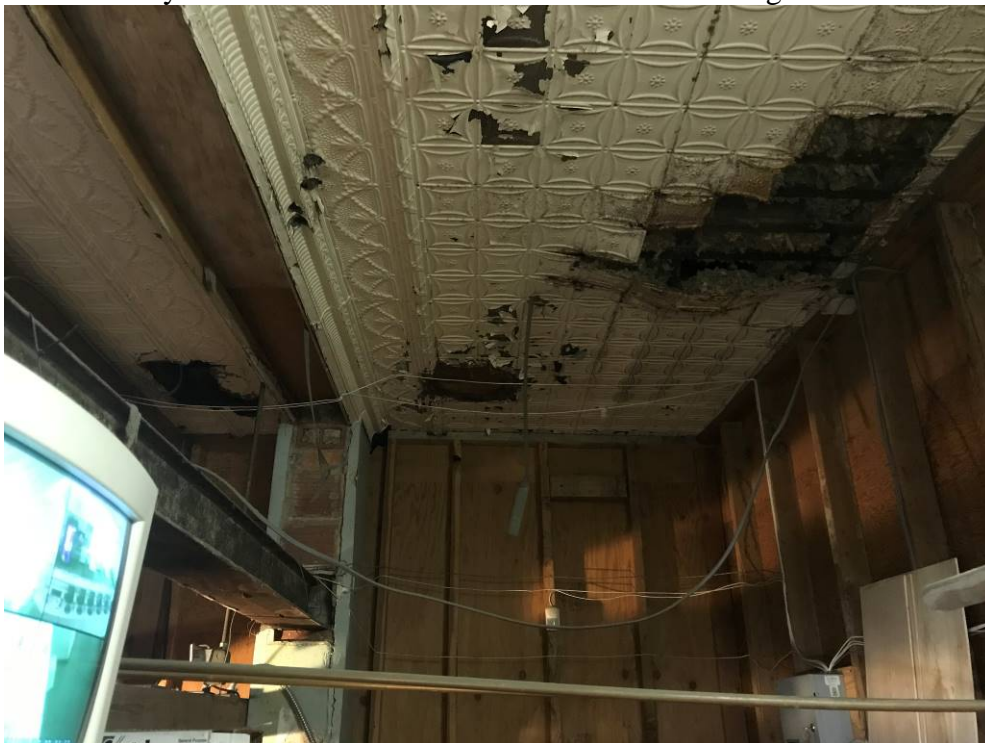
Photo 11: First Story Mechanical Space between West Area and East Area Looking North
