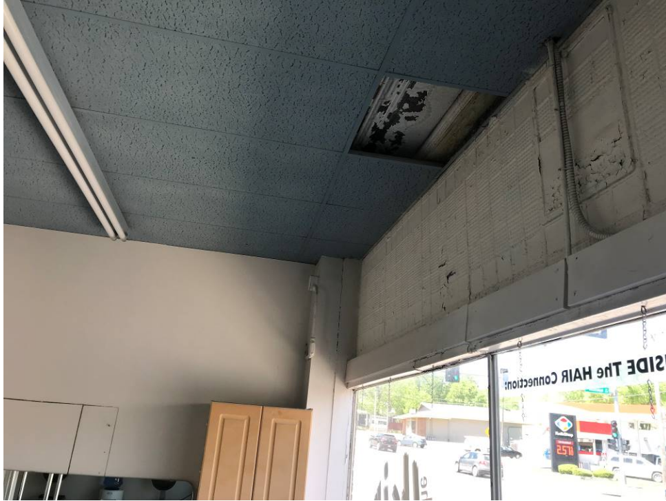
Photo 10: First Story Transom Over East Storefront and Tin Ceiling Above Modern Ceiling
