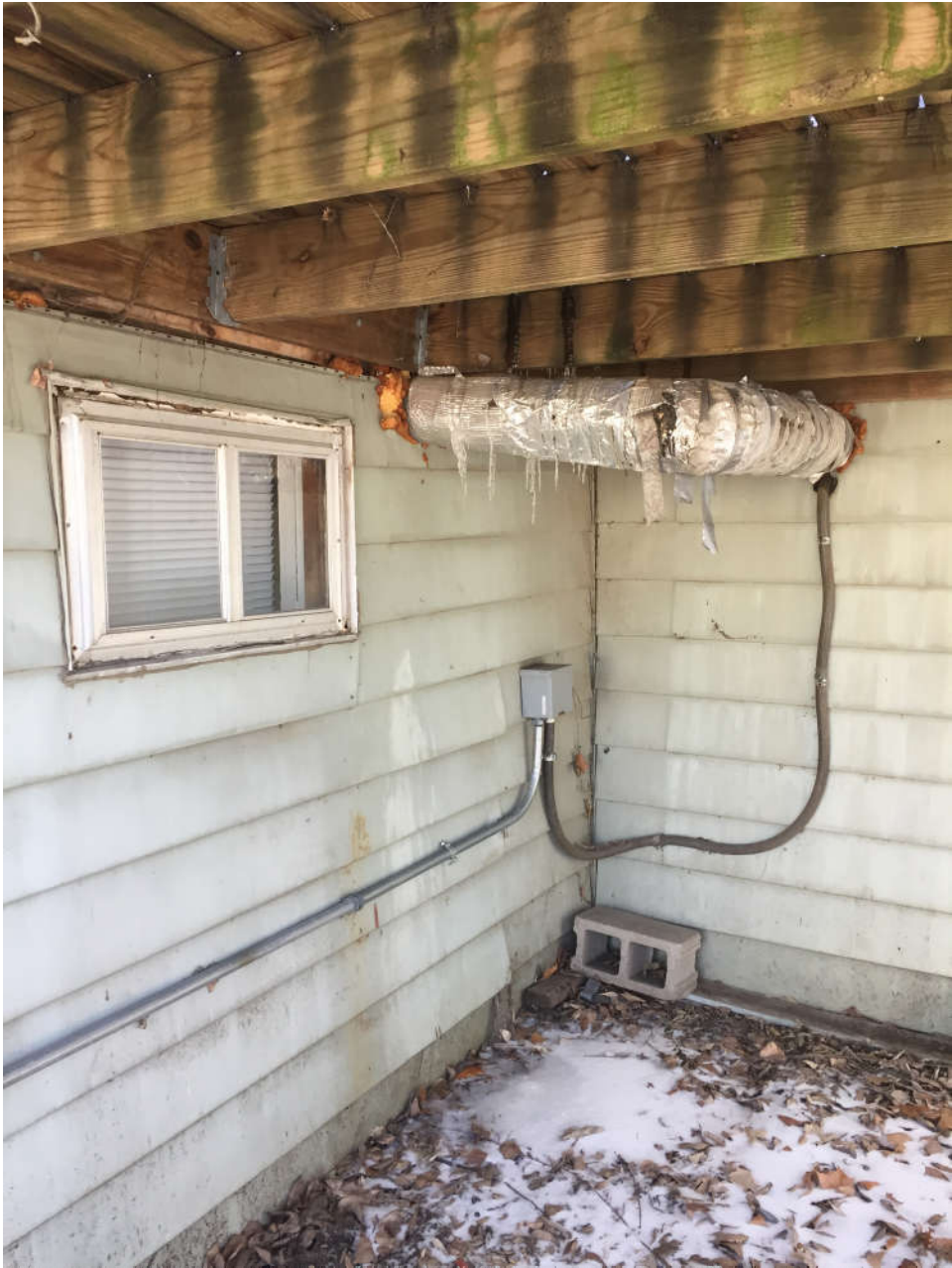
HVAC duct running through exterior walls.
