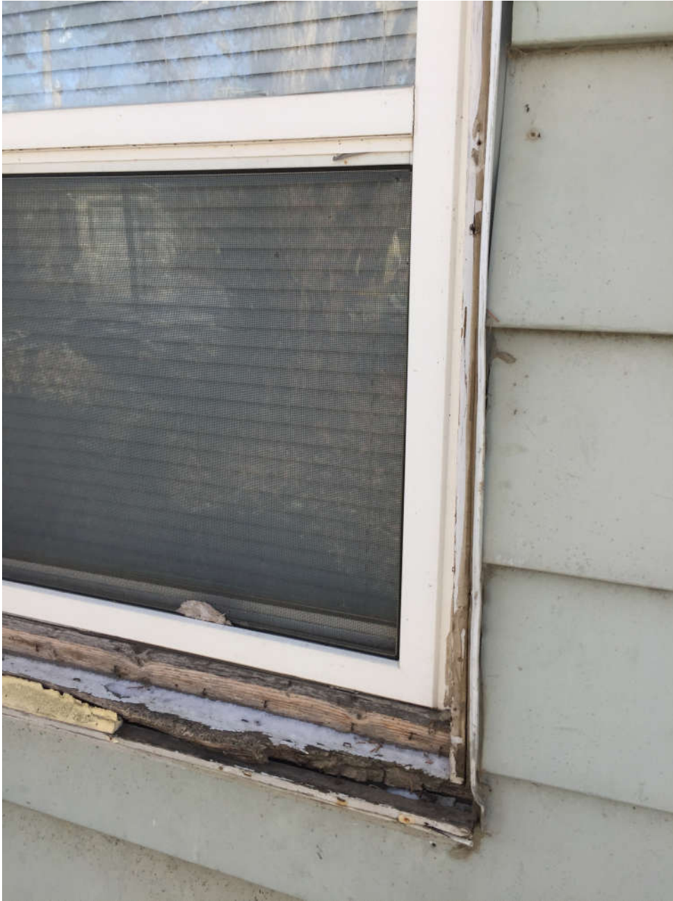
Window sill condition
