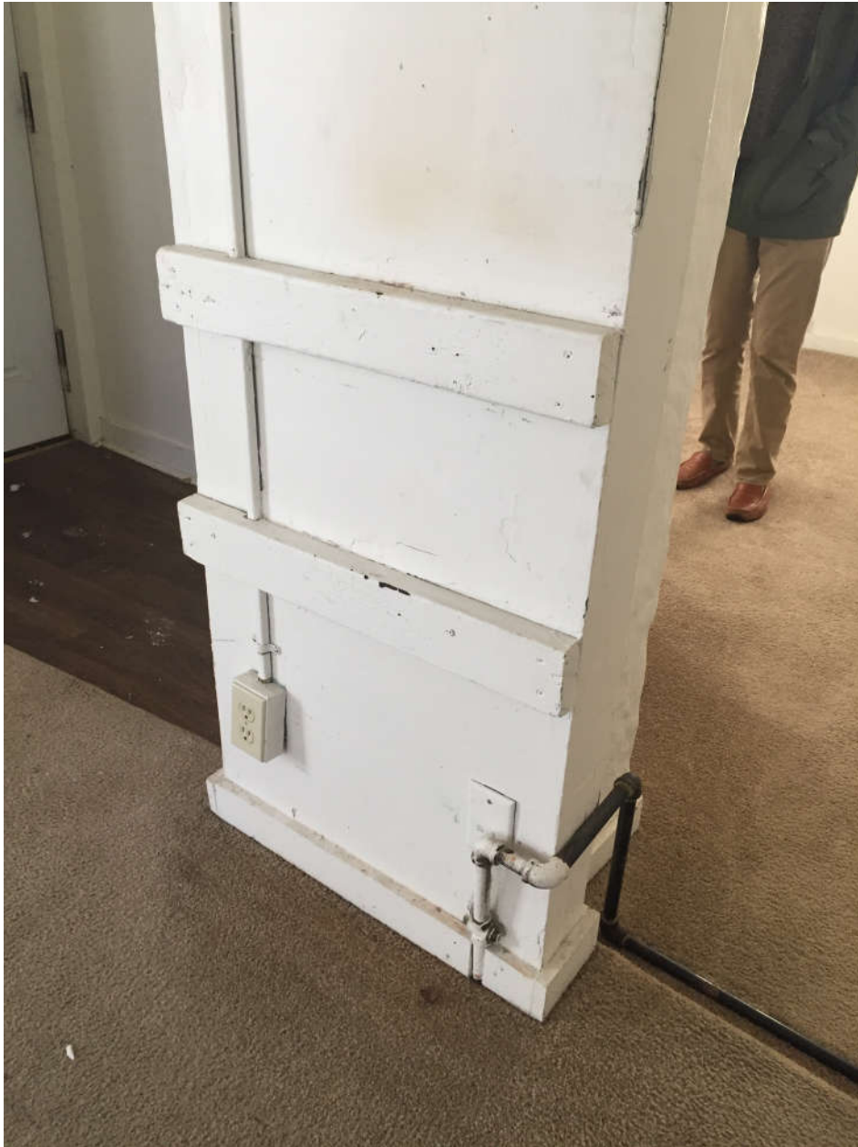
Sloping floors and exposed gas pipe
