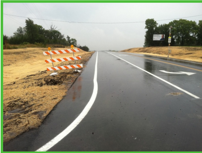
A new section of State Highway 56 includes a 4 foot paved shoulder in Baldwin, KS
