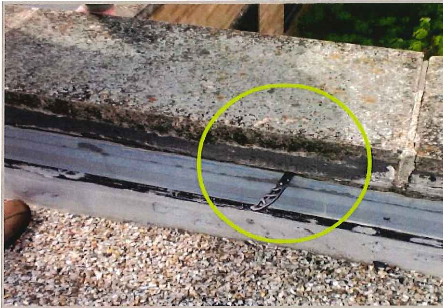
Area between the parapet wall and coping caps needs to be sealed to keep water from penetrating behind the flashings. This area shows where water is getting in behind the termination bar and under the roofing system.
