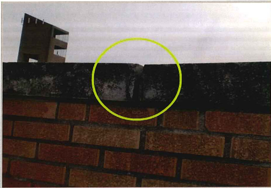
Joint on coping blocks do not have any sealant between the blocks.
