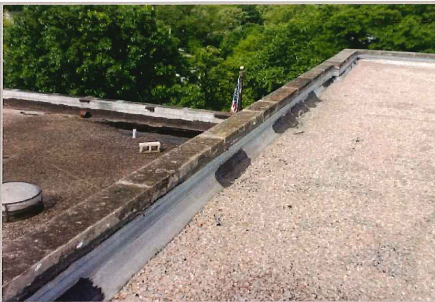
View of coping cap and flashing along Southwest corner of upper roof.
