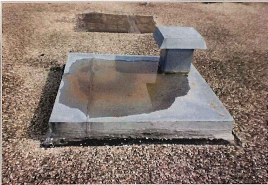
Flashings under the vents are in bad shape.
