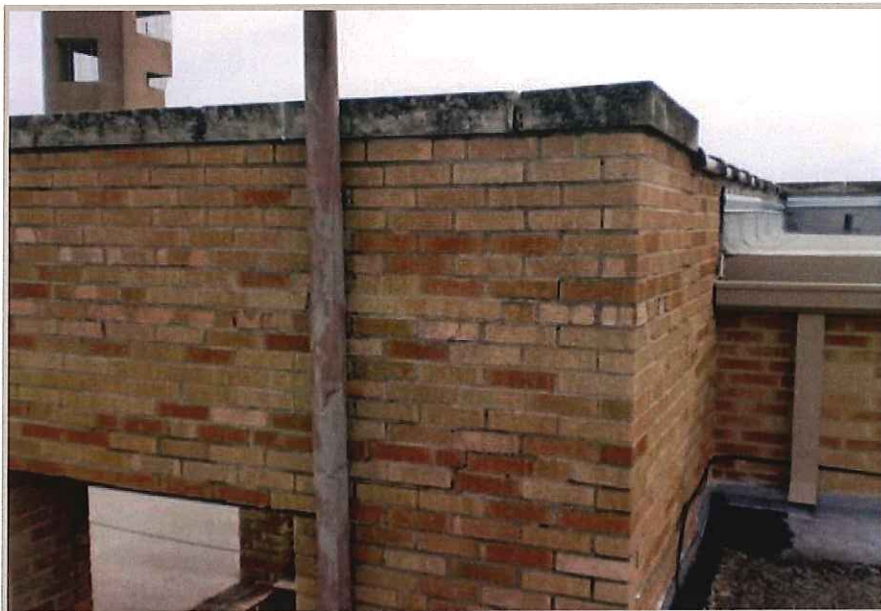
Bricks are flaking apart caused by water trying to evacuate the inside of the brick.
