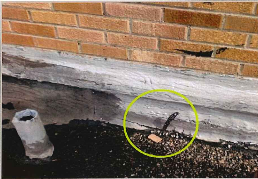
Flashing is cracked, allowing water in under the membrane.
