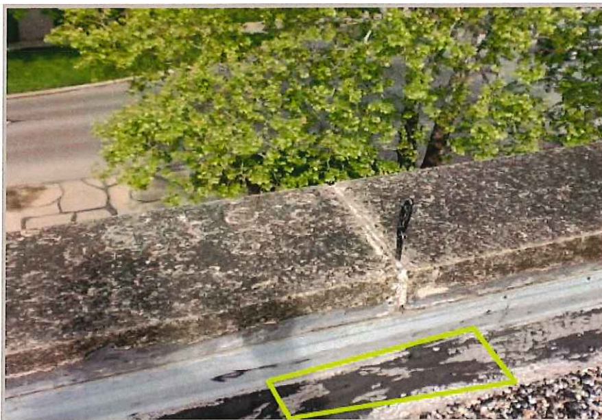
Base flashings appear to be made of Asbestos material. This will need to be checked in a lab to confirm.
