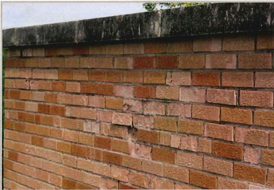
Bricks are flaking off the wall due to water standing inside the bricks. There needs to be a way for water to drain out to resolve this problem.
