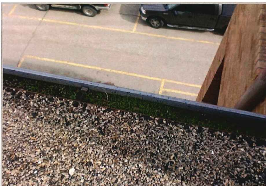
Gutters are full of gravel and grass. This should be cleaned out to keep water off the roof
