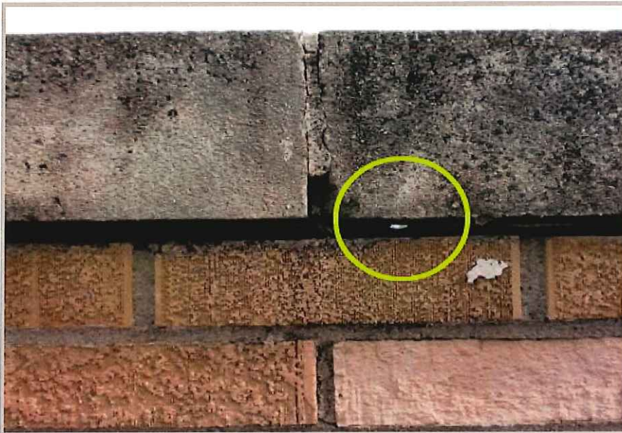
Daylight is showing under the bricks.
