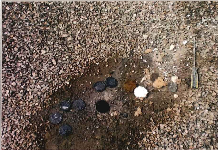
Core sample indicates there are 2 roofing systems on this facility. The roofing system under the Built up Roof with gravel is still in good shape and may be the reason the water is not penetrating the inside of the building.
