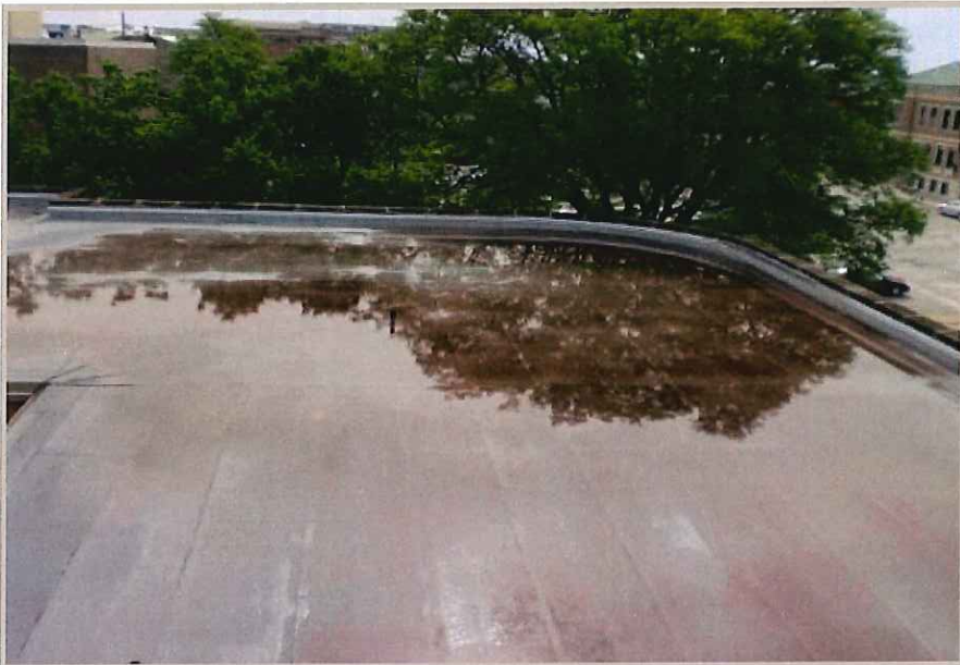
There should be a minimum of 2 Scuppers installed in the corner of this roof to allow water to drain.
