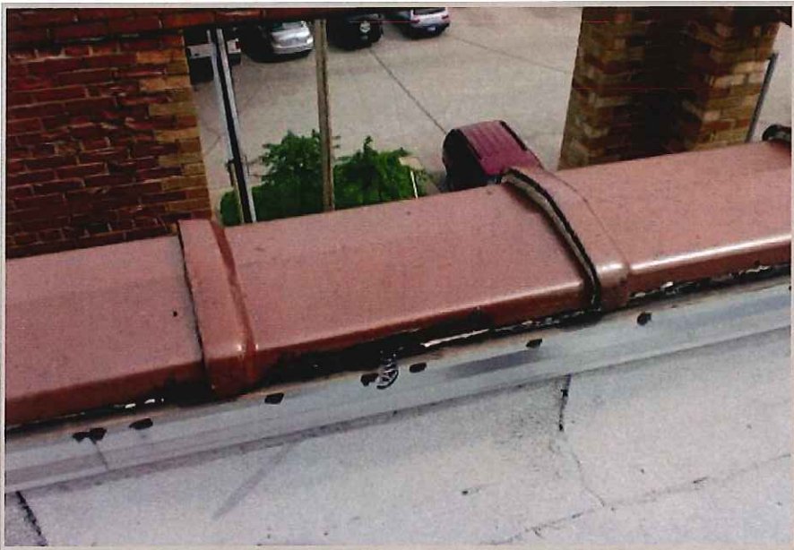
Poor repairs have been made on the Stone Coping Caps. Water is getting under the Stone Caps and draining inside the wall cavity.
