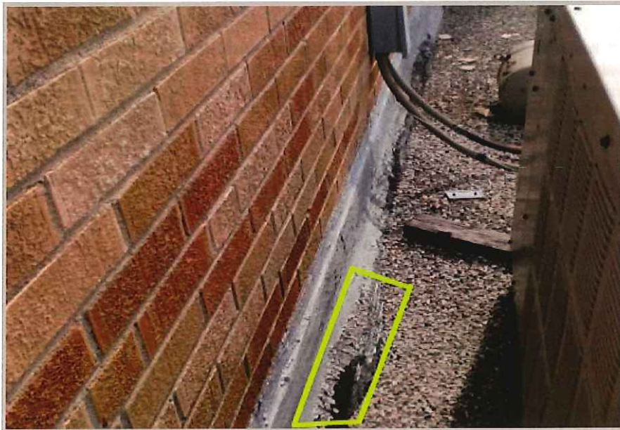
Flashings are pulling apart, scrim is exposed.
