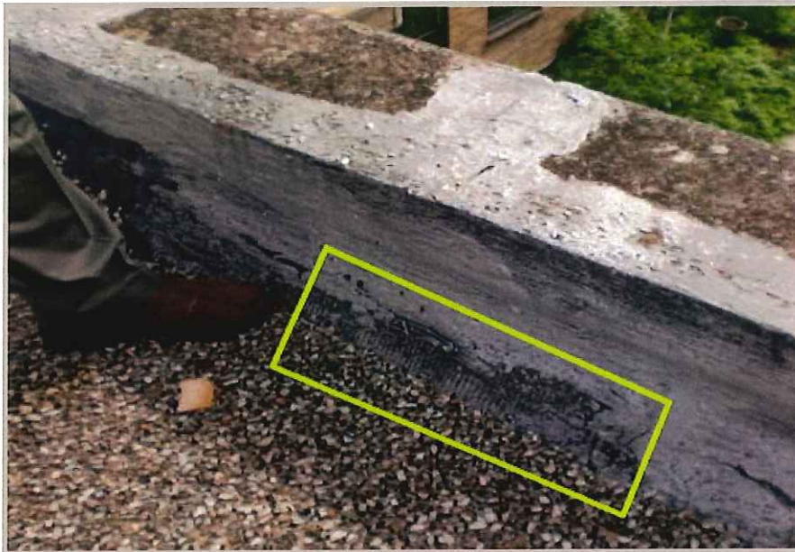
Membrane has worn away leaving the scrim exposed. UV rays are damaging to these types of areas.
