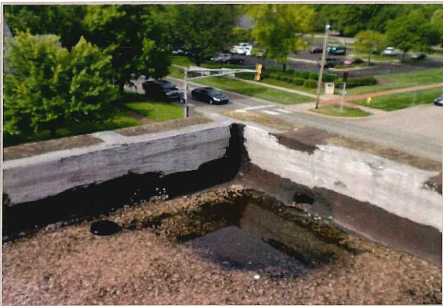
Southwest corner, water standing around scupper.
