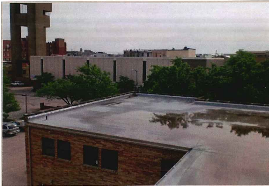
This roof has no drainage at all. All the water runs towards the Southeast corner with no where to go. The roofing system that has been installed on this facility is not designed to hold water and will only shorten the life of the system.
