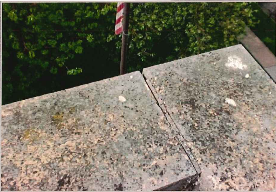
The joints on the stone coping caps are failing. Water gets between the blocks and runs into the brick wall as well as under the roofing system.
