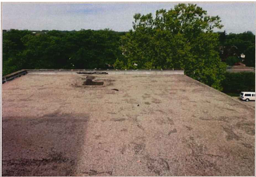
This section is covered with blisters to the extent you need to be carefull where you walk to keep from breaking the blisters open. Blisters are caused by moisture and gases under the membrane.
