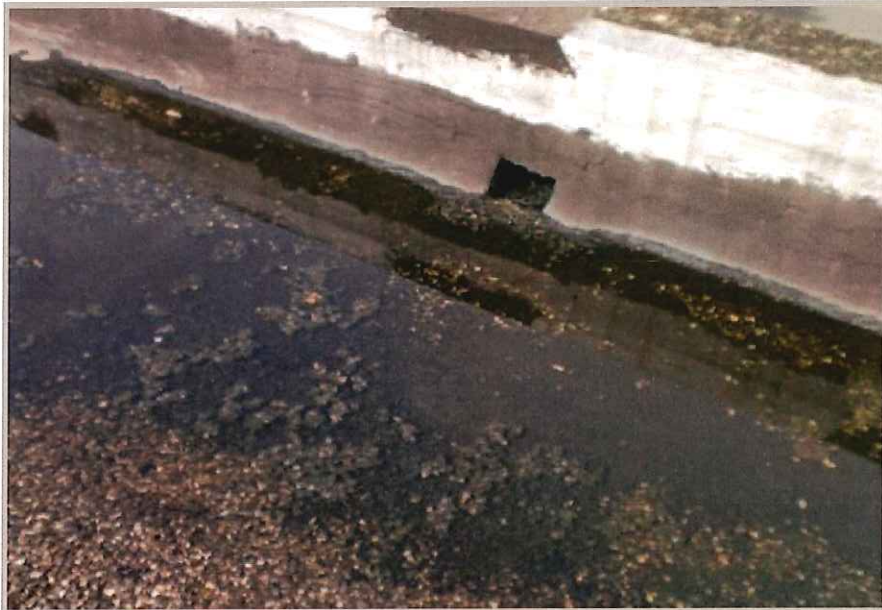
Flood and Gravel roofs are capable of holding some water although roof should drain better.
