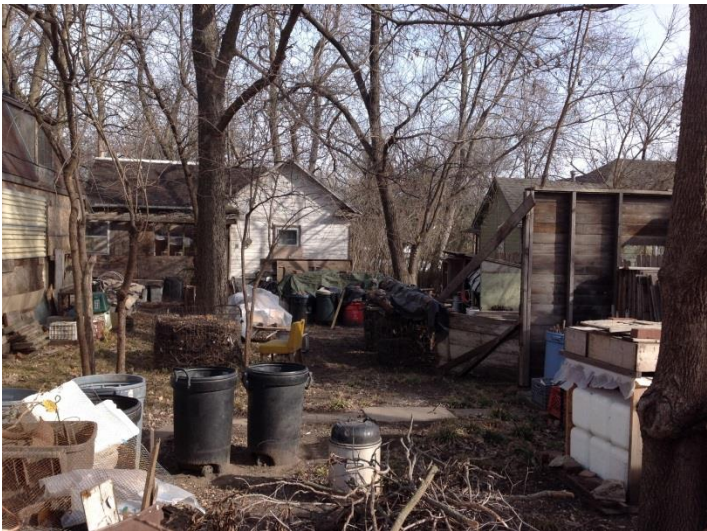
Storage/debris and accessory structure – only 3 sides standing
