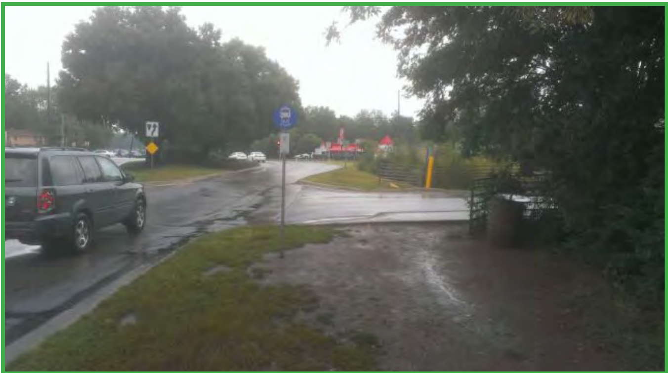
Figure 5-18: Naismith Drive – Bus Stop with No Concrete Pad.
