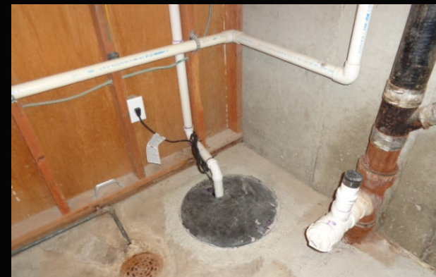
New Sump Pump Discharging Outside
