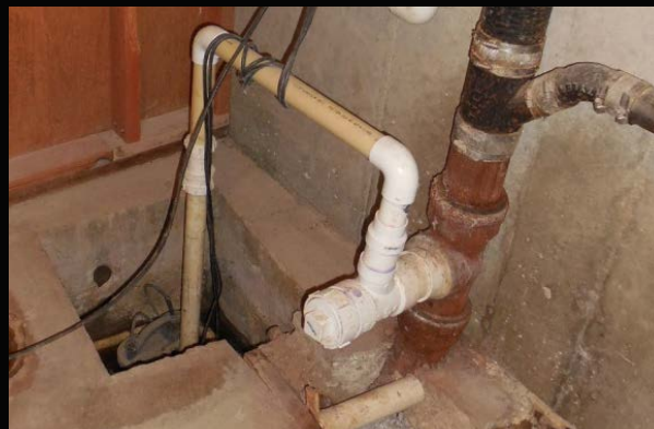
Sump Pump Connected to Sanitary Sewer
