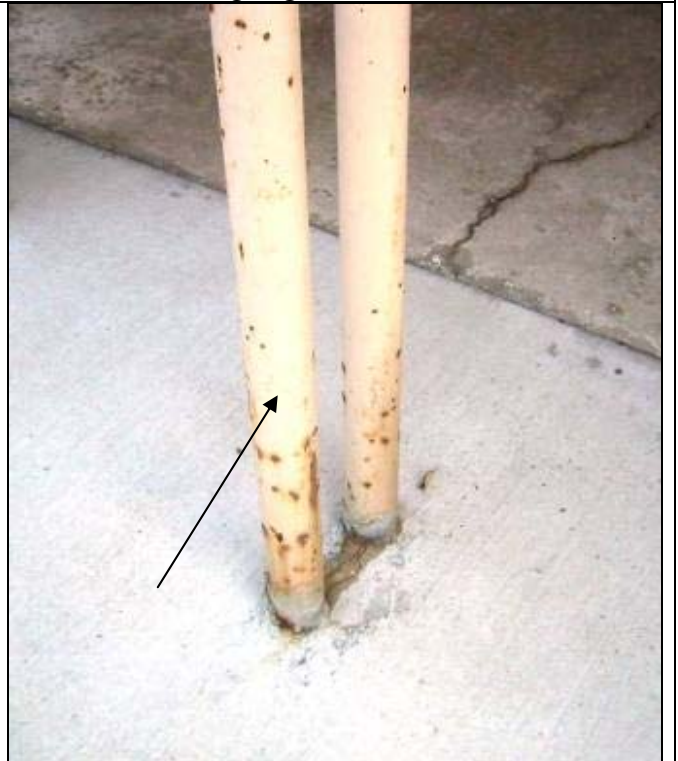
Deteriorated LBP on the exterior columns
