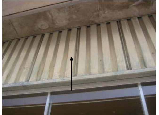
Deteriorated LBP on the exterior A wall siding
