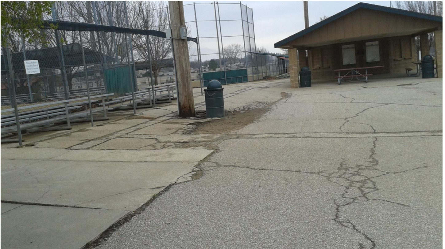
Holcom Complex – Replace damaged asphalt inside complex $35,000
