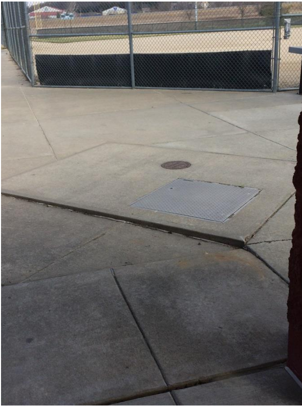
Clinton Lake Softball Complex – replace damaged concrete inside complex $20,000
