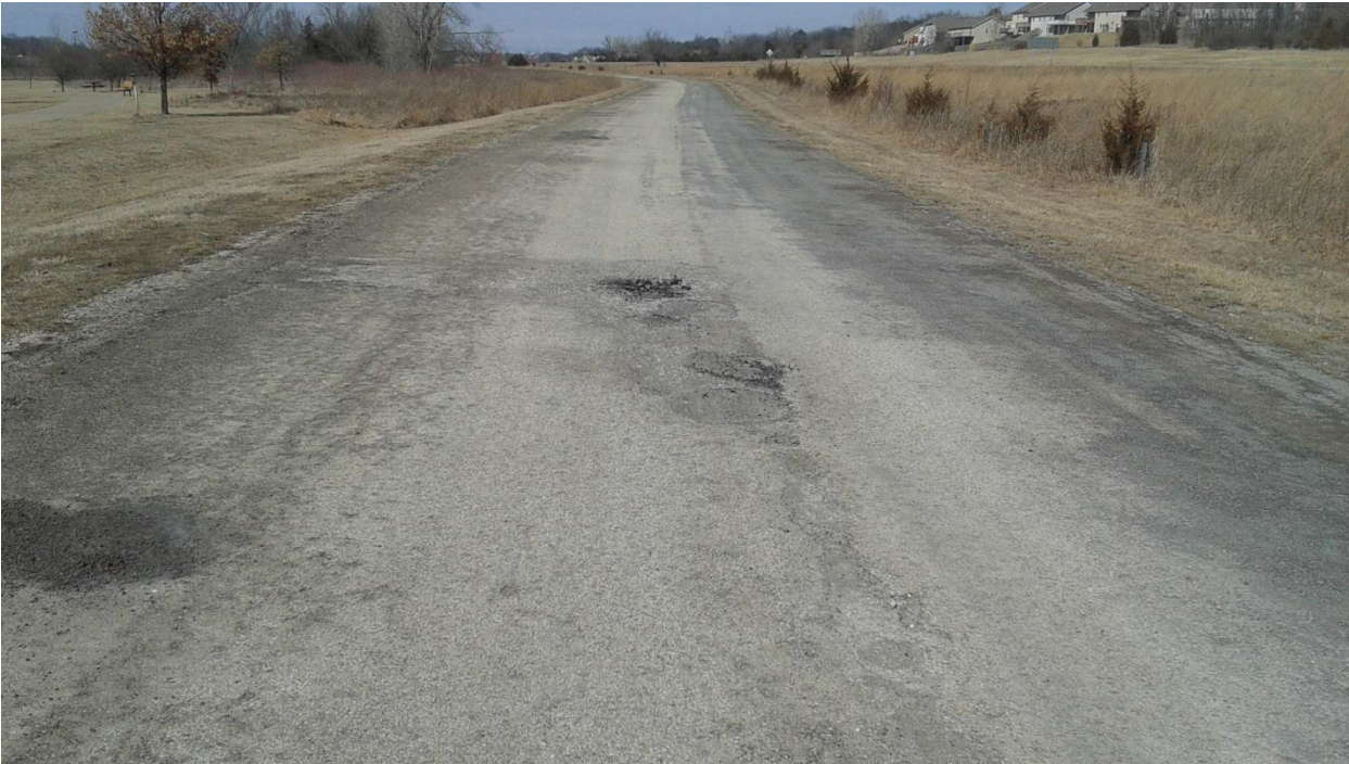
Clinton Lake Softball Complex - Speicher Road to the complex– Patch / Chip & Seal $45,000
