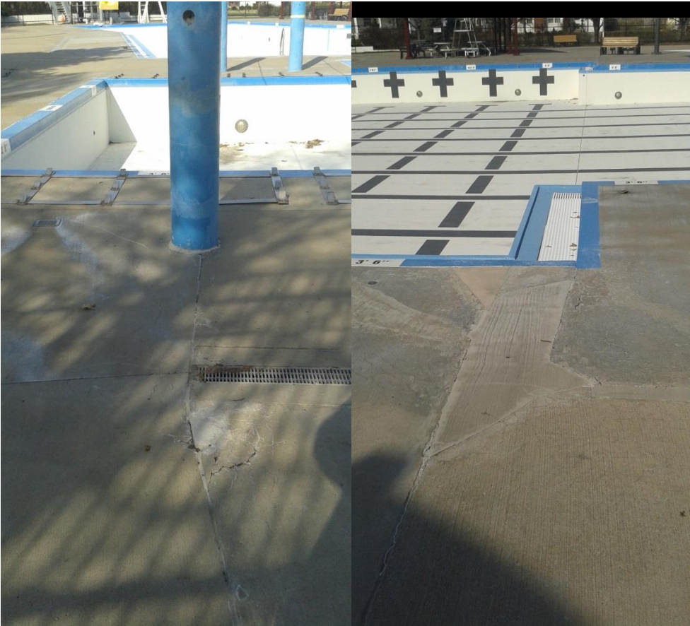
Outdoor Aquatic Center Remove and replace bad sections of pool deck $85,000
