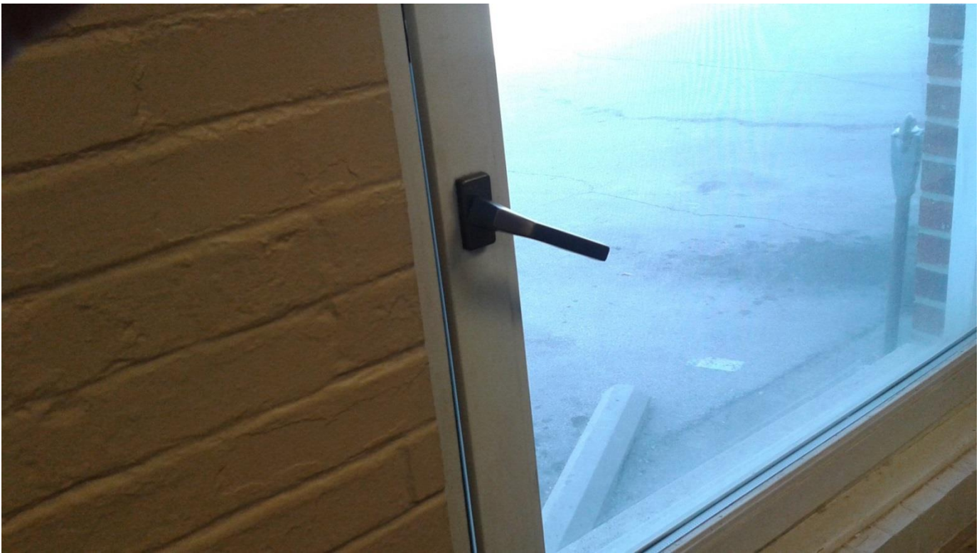
Community Building – Replace windows that do not properly seal $35,000
