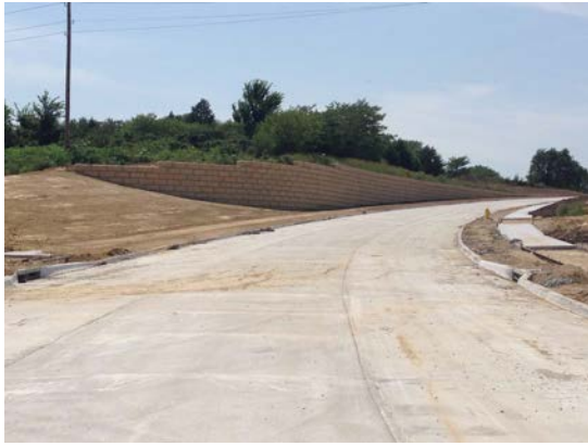
Venture Park infrastructure
