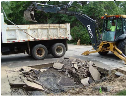
Crescent Road Sinkhole
