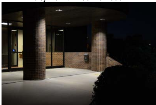
LED lighting at City Hall entry
