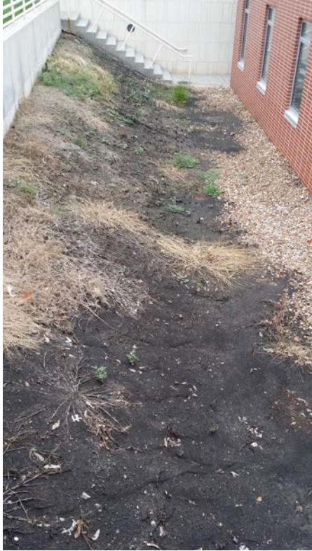
Drainage problem at Fire Station 5
