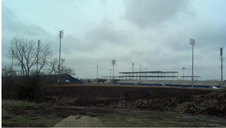
November 22, 2013, photo by Public Works staff
