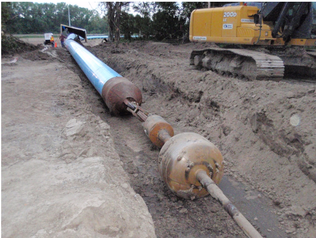
Looking west at 36" diameter fusible PVC pipe string and pulling head ready at the entry pit.
