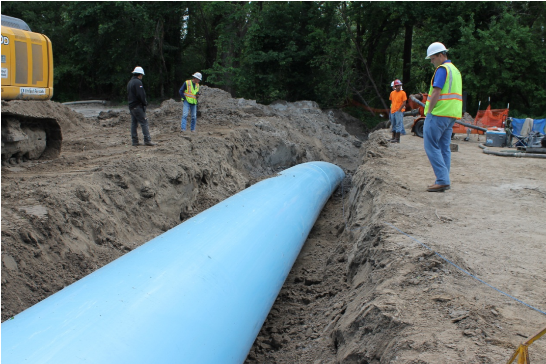
Pipe being pulled into the entry pit on the West side of the Kansas River.
