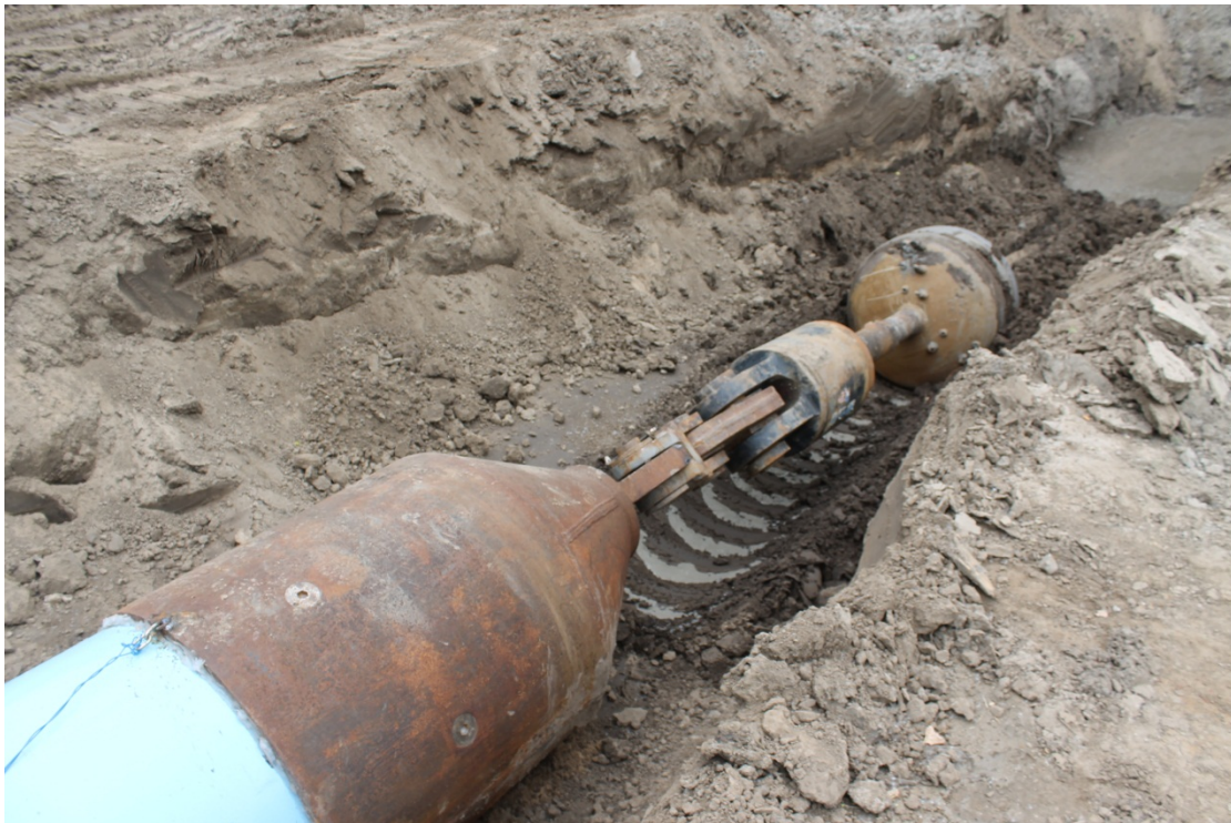
36" diameter fusible PVC pipe and pulling head ready at the entry pit.
