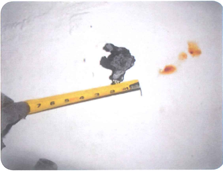
Paint Blistering Off Interior Walls
