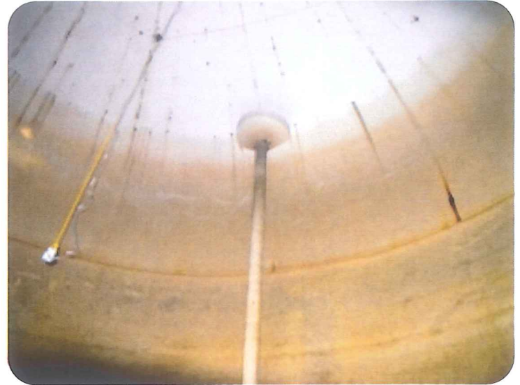
Rust Spots on Ceiling of Tank
