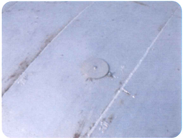
Exterior Coating on Top of Tank/Rust/Cathodic Plates that need to be Welded Shut due to Gaps
