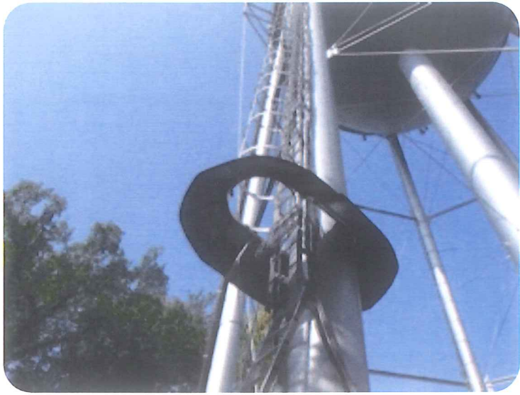
Ladder Cage & Lockable Cover on the Cage
