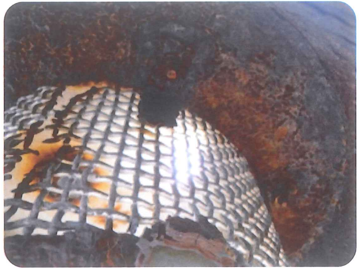
Underneath Vent & Vent Screen Corroded with Rust
