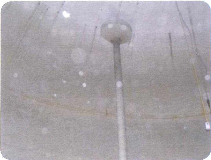
Rust Spots on Ceiling of Tank
