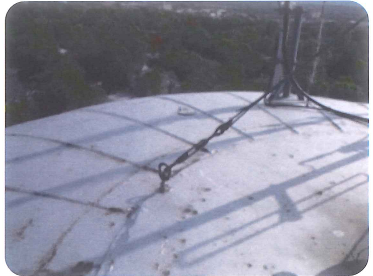
Exterior Coating on Top of Tank Peeling off & Rust Present
