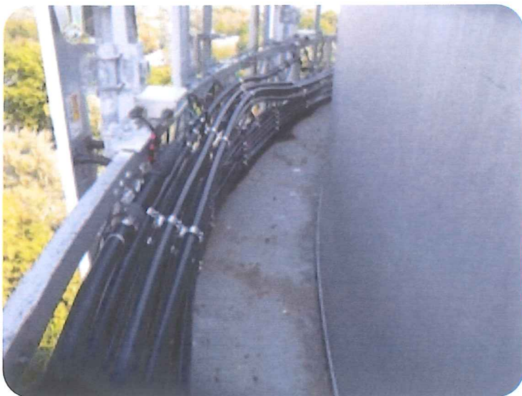
Coax Cables on Catwalk
