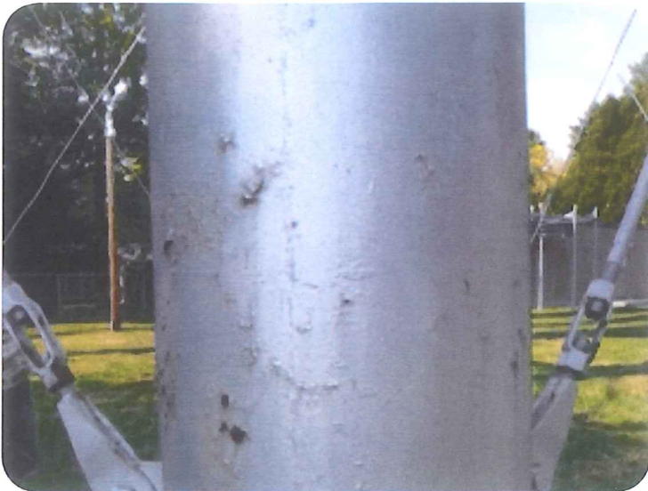
Exterior Coating Peeling off & Rust Present
