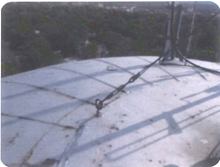
Rooftop Surface with Paint Deteriorating & Rust Present
