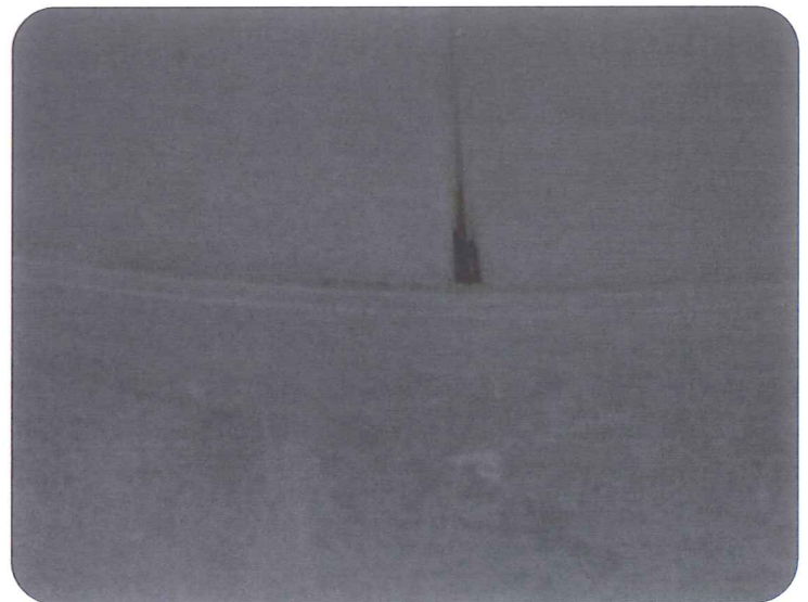
Rust Spot on the Interior of the Tank
