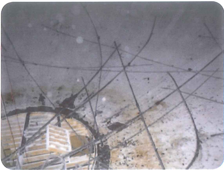
Bottom of Wet Bowl, Rust on Surface of Tank, & Broken Cathodic Rods that we Cleaned Out
