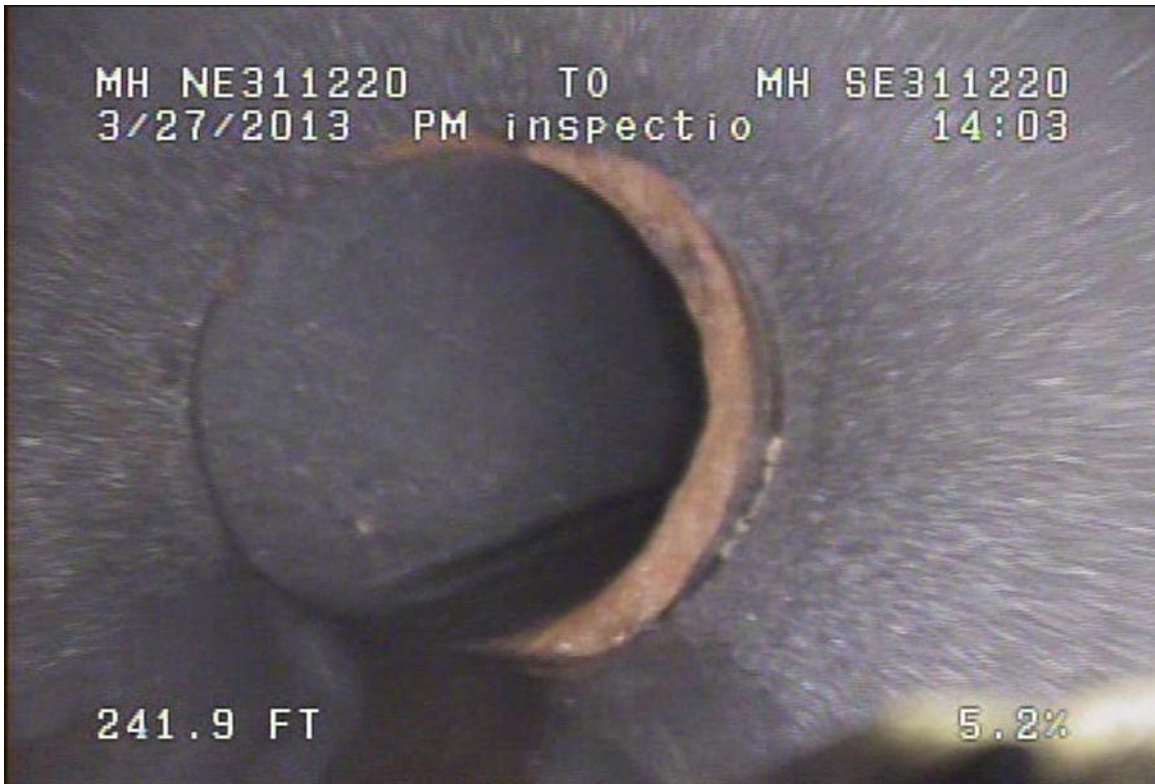
Photo below: Jog in pipe, turns right. No manhole
