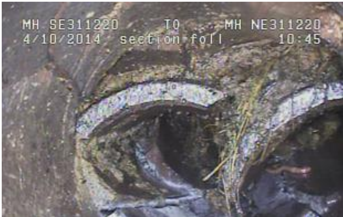
Photo below: Collapsed 8 inch city sewer main
