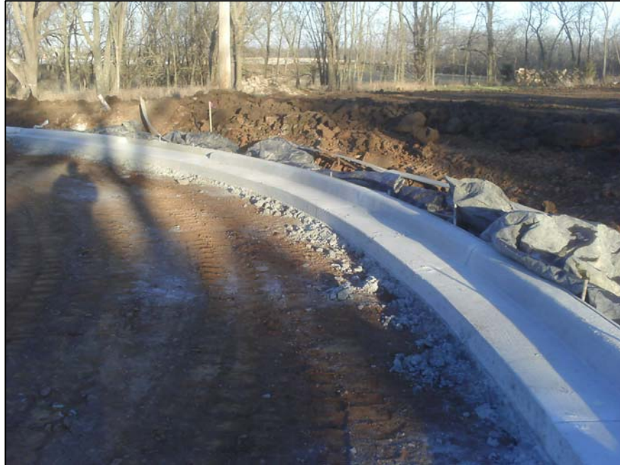
No tie bars. Requested Contractor install epoxy coated bar to be drilled and grouted.
