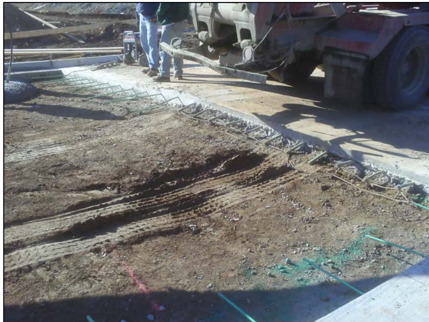
Backed ready-mix truck over dowel bars. Note deformed tie bars in Left Lane.
