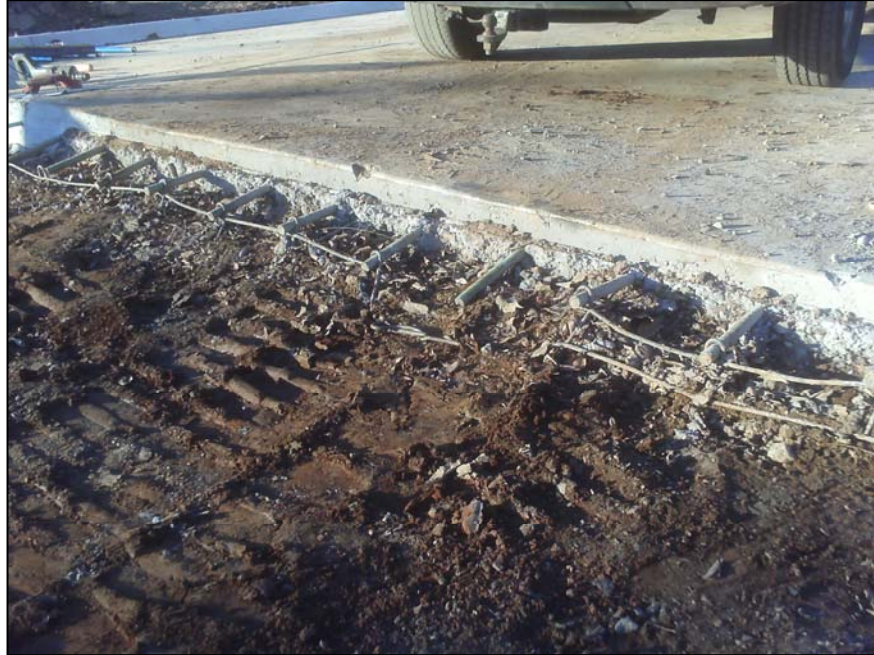
Bent dowel bars.
