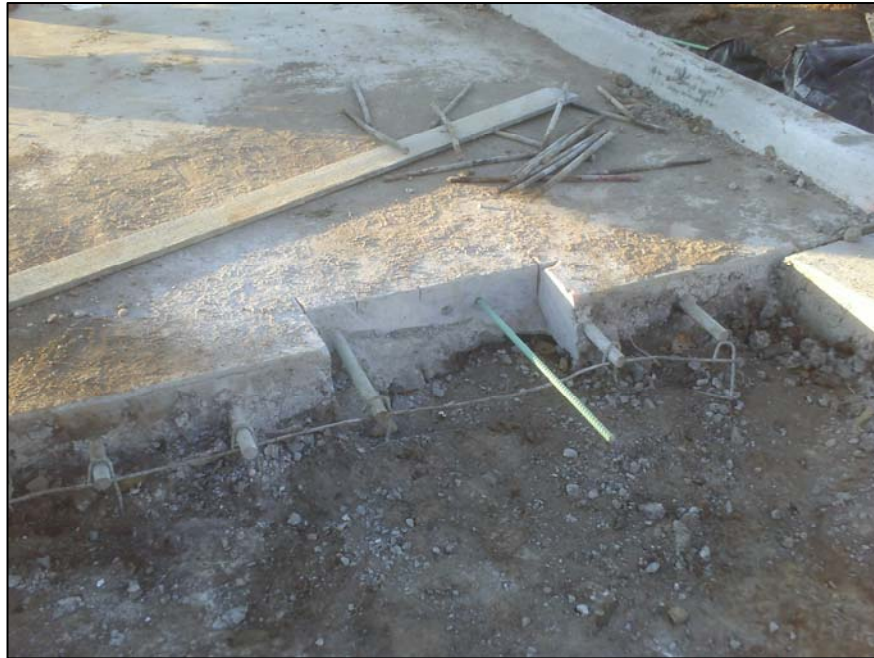
Construction joint on George Williams Way.
