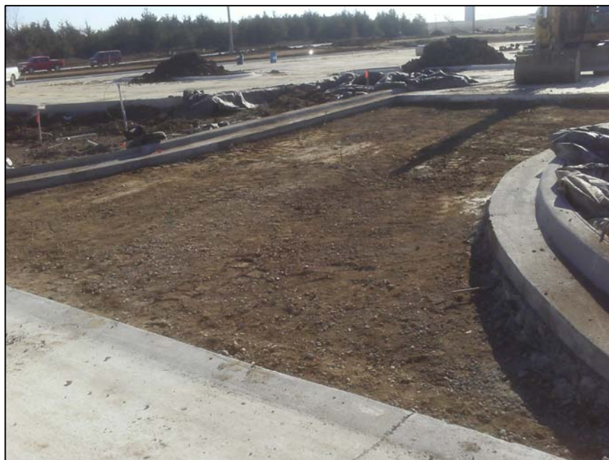
Private Drive to Parking Lot Entrance No tie bars to Curb and gutter.
