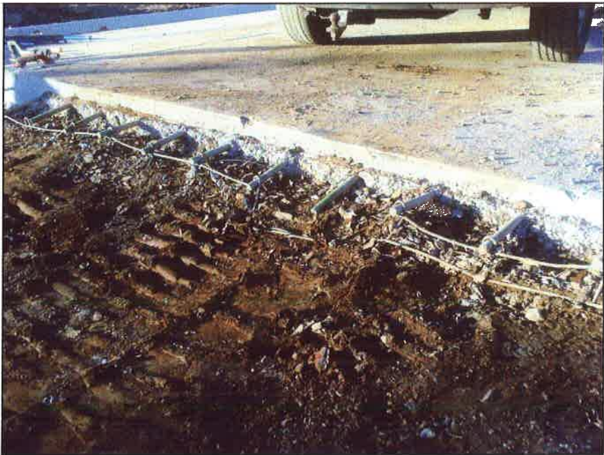
Bent dowel bars.
