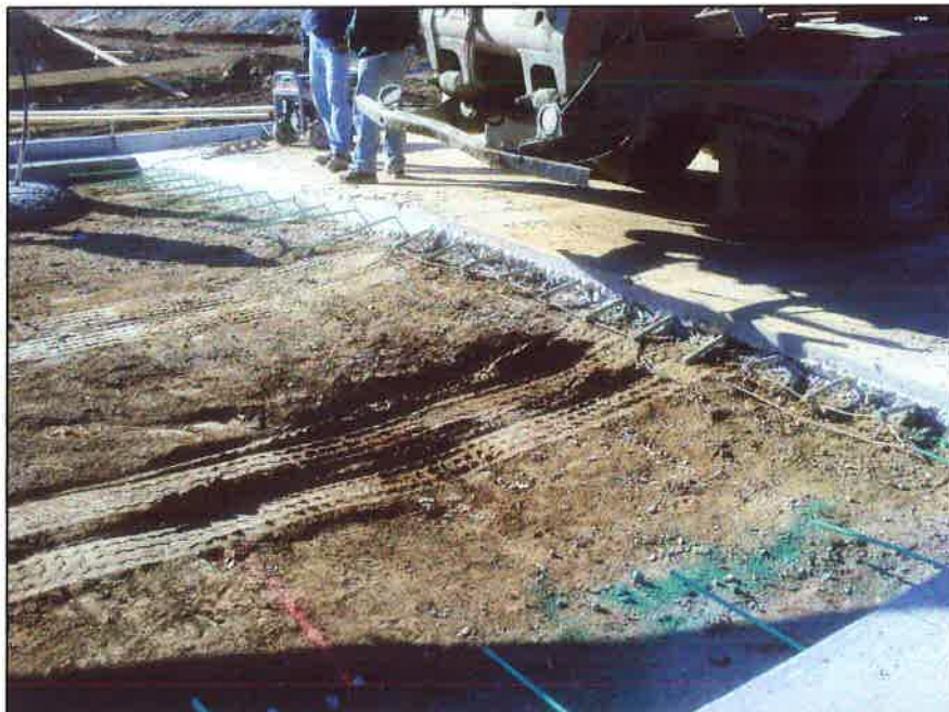
Backed ready-mix truck over dowel bars. Note deformed tie bars in Left Lane.
