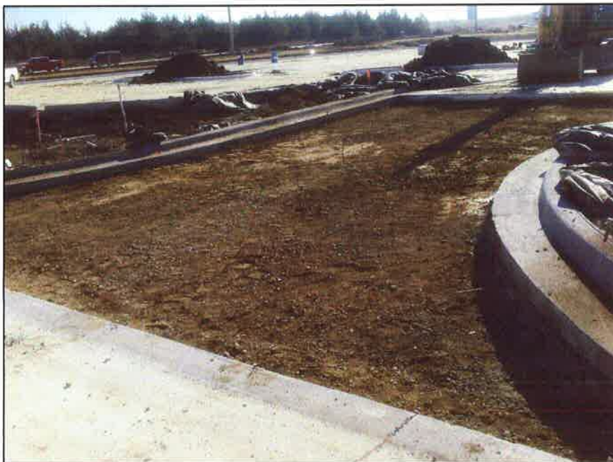
Private Drive to Parking Lot Entrance No tie bars to Curb and gutter.
