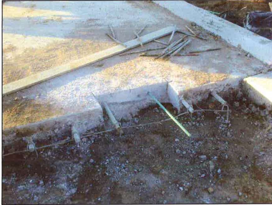
Construction joint on George Williams Way.
