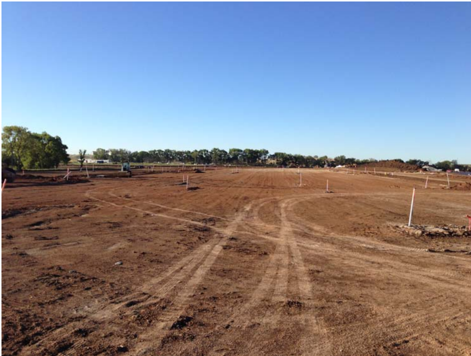
Irrigation conduit sticking out of future parking lot islands
