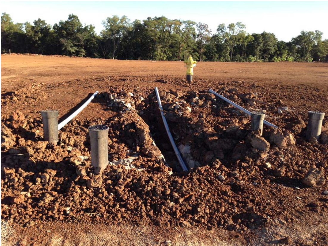
Fire hydrant and water valves
