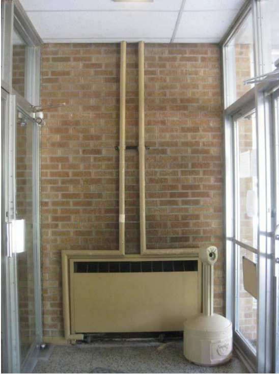
Air handler waiting room by south entrance 16September2009
