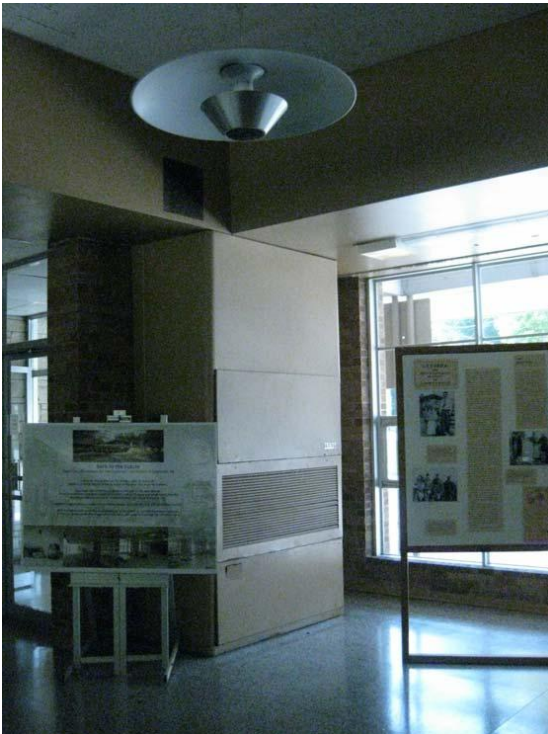
Fan coil in southern vestibule 16September2009
