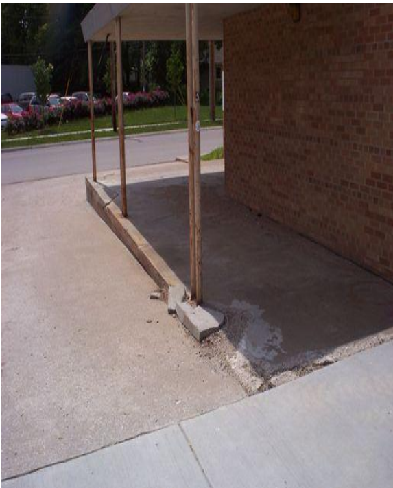
Sidewalks need repairing on and near south side of the building 04MAY2012
