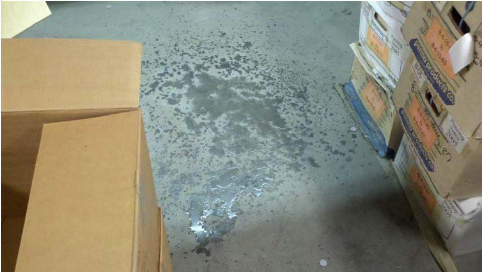
A leaking ceiling at SWAN compromised the long term survival of some records.
