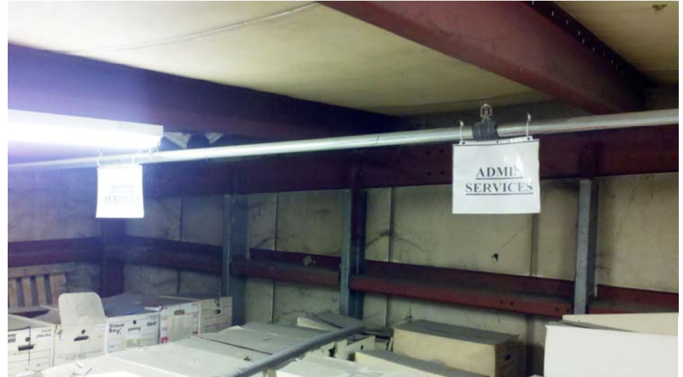
Fire sprinklers at SWAN protected the building, but threatened the records.
