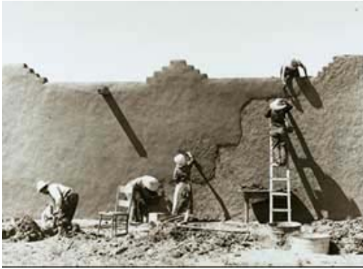
Traditionally, adobe surface coatings that protected the fragile adobe building fabric were renewed every few years. Women are seen here recoating an adobe wall with mud plaster mixed with straw at Chamisal, New Mexico. Photo: Russell Lee, Farm Security Administration Collection, Library of Congress.
