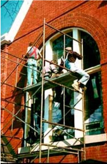
These workmen are performing exterior window maintenance after the protective glazing--which had prevented maintenance--was removed. Photo: Neal A. Vogel.
