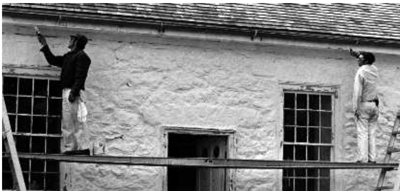
Adequate protection and maintenance of a historic building is an ongoing commitment. Here, two workers are priming and repainting exterior stone and wood trim. If surface treatments are neglected, more extensive repair and replacement will be required. Each loss further undermines a building's historic integrity. Photo: NPS files.
