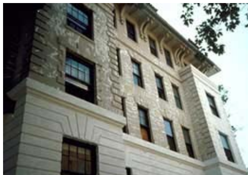
The caulking shown here is not an appropriate method for repairing cracks in historic stucco. Photo: NPS files.
