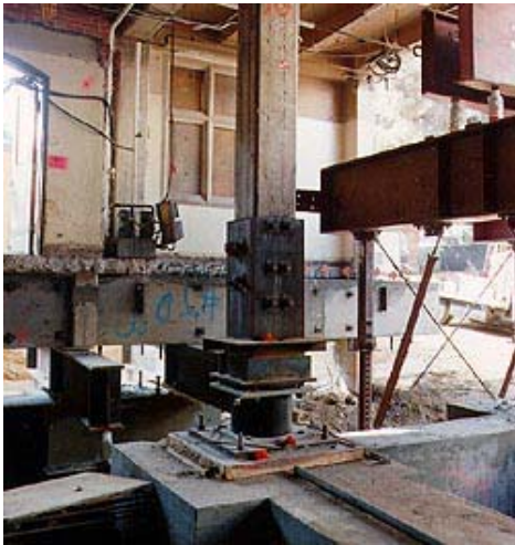
The new base isolator allows the structural support member at the foundation to move horizontally as it absorbs the earthquake forces. Photo: ©Jonathan Farrer.
