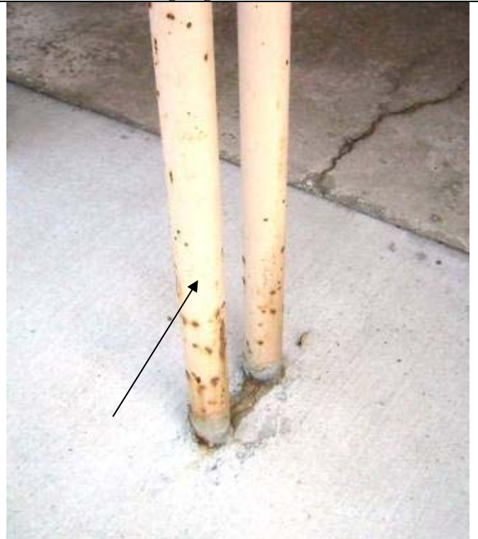
Deteriorated LBP on the exterior columns
