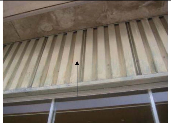
Deteriorated LBP on the exterior A wall siding
