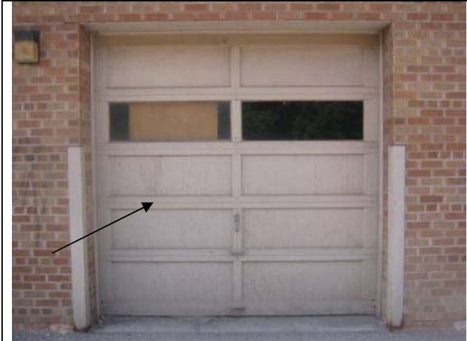
Deteriorated LBP on the exterior C wall garage door face.
