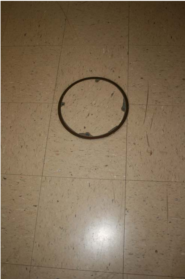
File Name : WireChaseCoverInFloor.JPG Shooting Date/Time : 9/16/2009 10:28:07 AM
