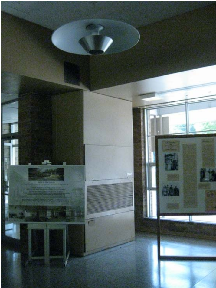
File Name : AirhandlerWaitingRoom.jpg Shooting Date/Time : 9/16/2009 12:21:26 PM
