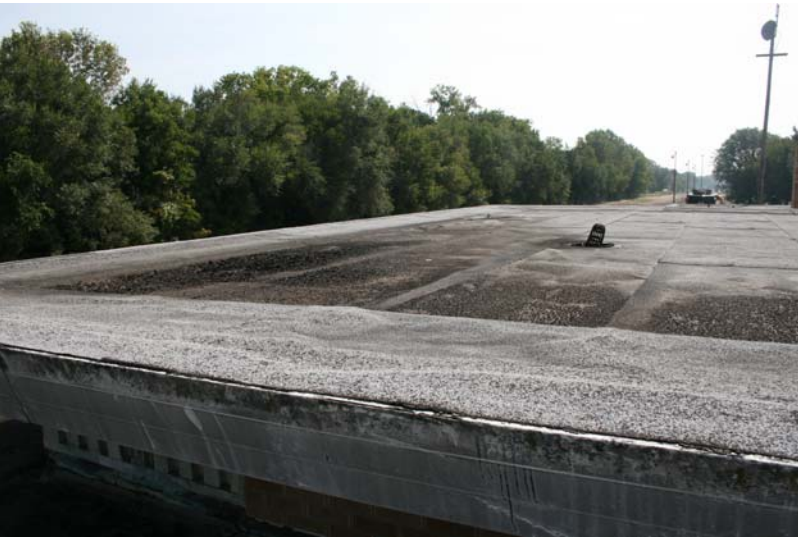
File Name : RoofWornOut1.JPG Shooting Date/Time : 9/16/2009 11:27:51 AM
