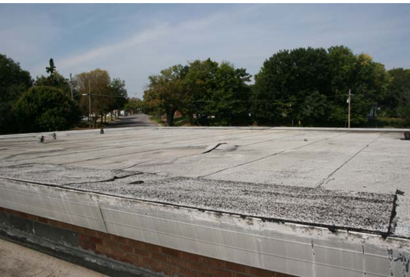
File Name : RoofBlister2.JPG Shooting Date/Time : 9/16/2009 11:32:02 AM
