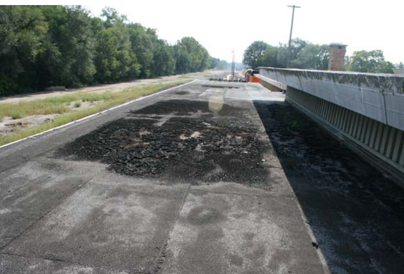
File Name : RoofWornOut2.JPG Shooting Date/Time : 9/16/2009 11:27:24 AM
