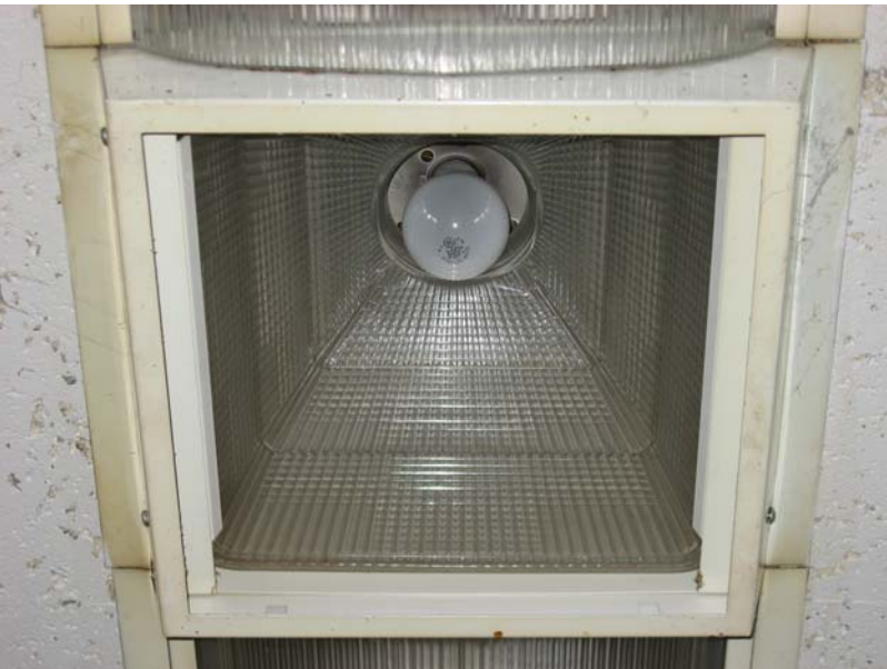
File Name : LightFixtLensMissing.JPG Shooting Date/Time : 11/9/2009 3:34:21 PM
