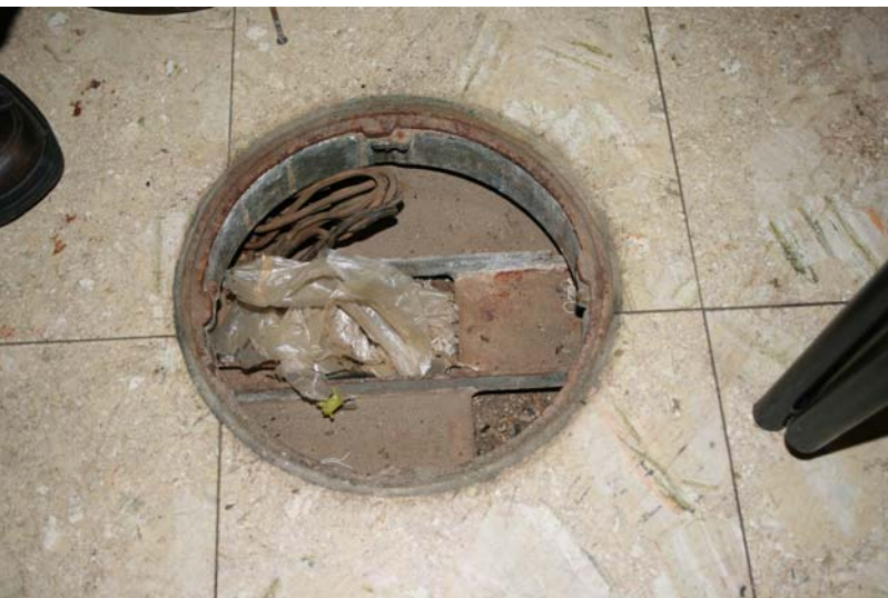
File Name : WireChaseOpenInFloor.JPG Shooting Date/Time : 9/16/2009 10:57:20 AM
