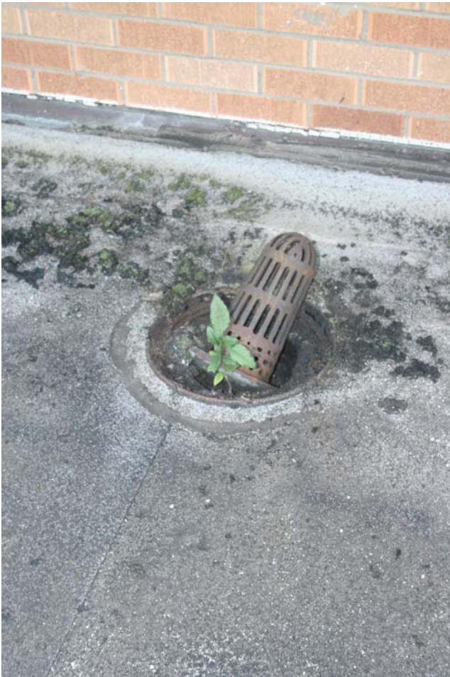
File Name : RoofDrain.JPG Shooting Date/Time : 9/16/2009 11:27:47 AM
