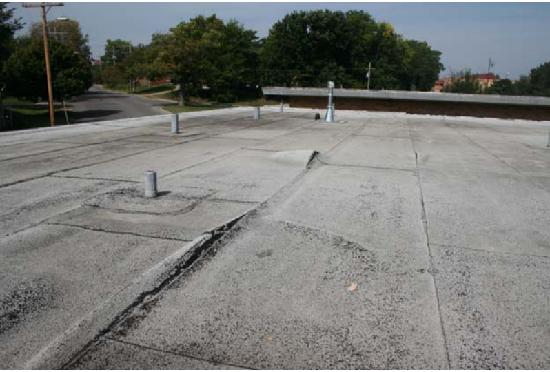
File Name : RoofBlister1.JPG Shooting Date/Time : 9/16/2009 11:35:28 AM
